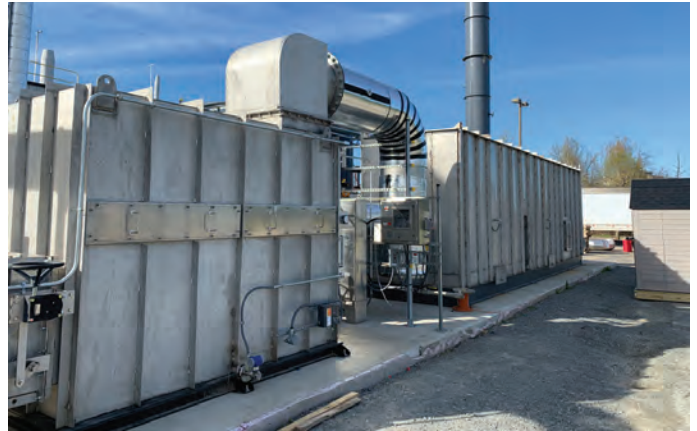
Food Processing Wastewater System Odor Control
