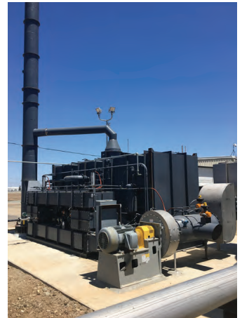
Asphalt Terminal Odor Control
