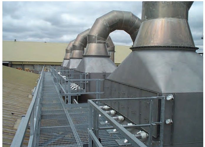
Granulator Scrubber Mist Elimination
