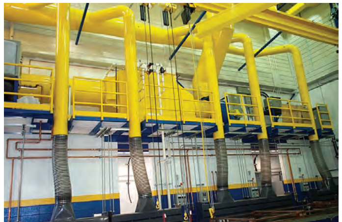
Wet Scrubber with Crossflow Hoods
