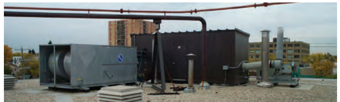
Condensing Crossflow Wet Scrubber Odor Control System
