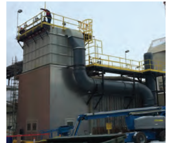
Nickel Dust Collector
