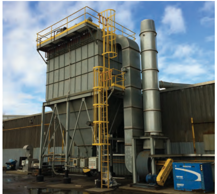
Baghouse Dust Collector
