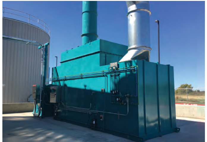
Roofing Plant Mist Collection System
