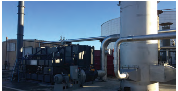
Asphalt Terminal Odor Control
