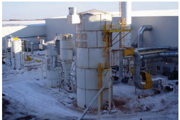
Dust Collection and Pneumatic Conveyance
