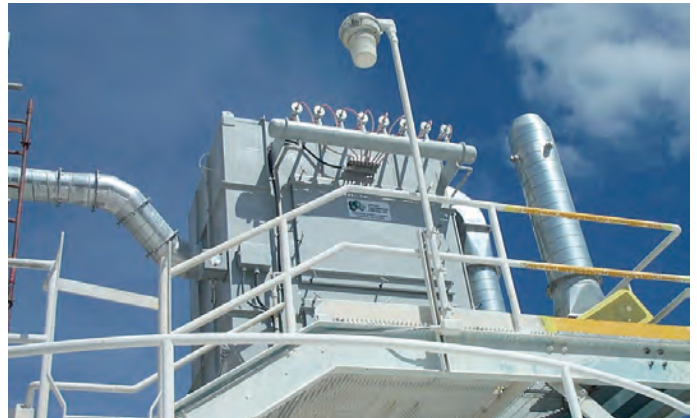
Lime Silo Venting Dust Collection System
