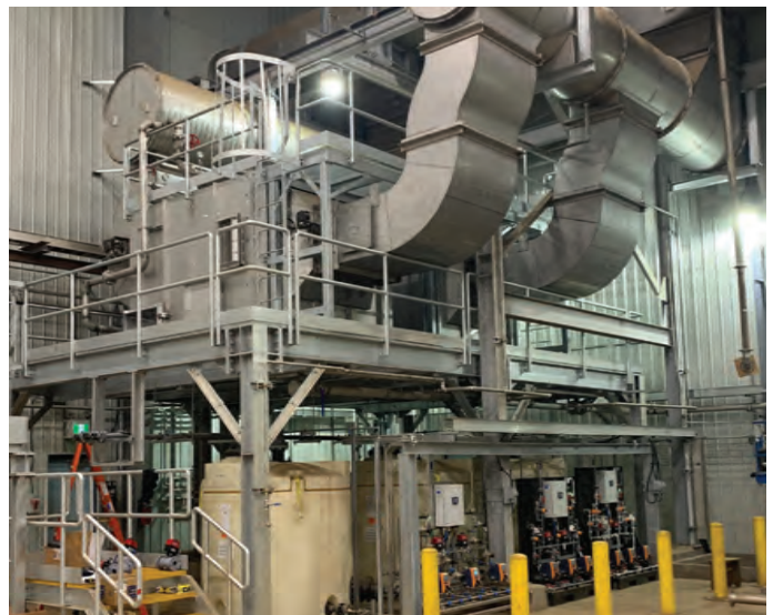
HSADF Wet Scrubber – Chemical Feed System
