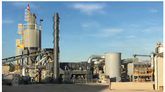
Hot Mix Plant Odor Control
