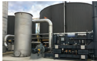
Asphalt Terminal Odor Control
