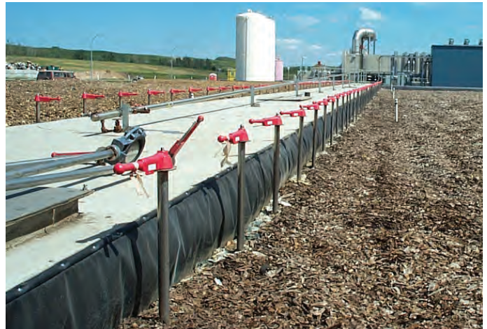
Open Top Biofiltration System
