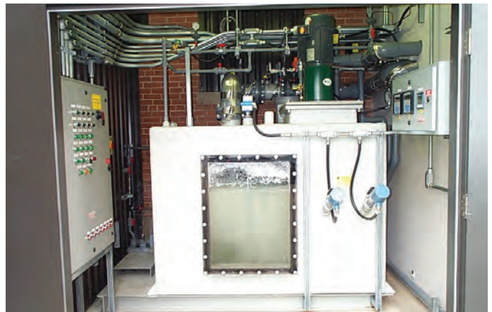
Remote Scrubber Sump
