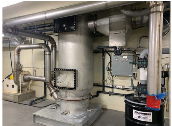
Water Treatment System SBS Scrubber
