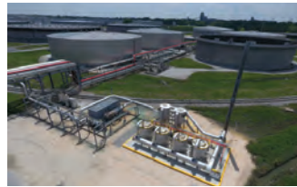
Asphalt Refinery Odor Control
